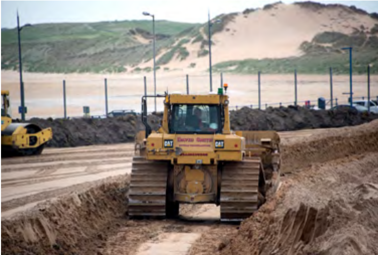
Digging deep! Work progresses on the largest LEADER grant funded project in Aberdeenshire to date – Fraserburgh South Links Sports Development Trust
