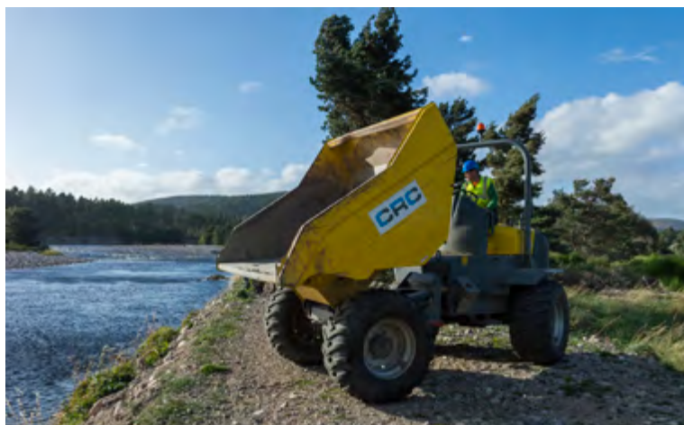
Ballater Flood Protection Works, September 2016 Flood protection forms part of climate change adaptation work
