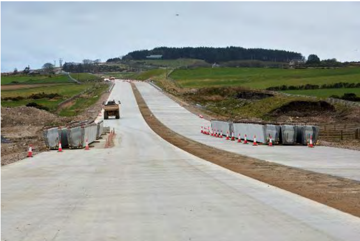
The AWPR/B-T is the longest roads construction project in the UK at 58 kilometres
